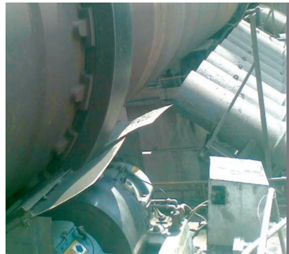
Reliability of the kilns has improved with the implementation of Mobil SHC 639
